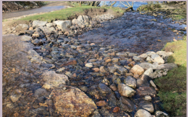
Stream crossing improvement on South Loch Ness Trail between Whitebridge and Foyers
