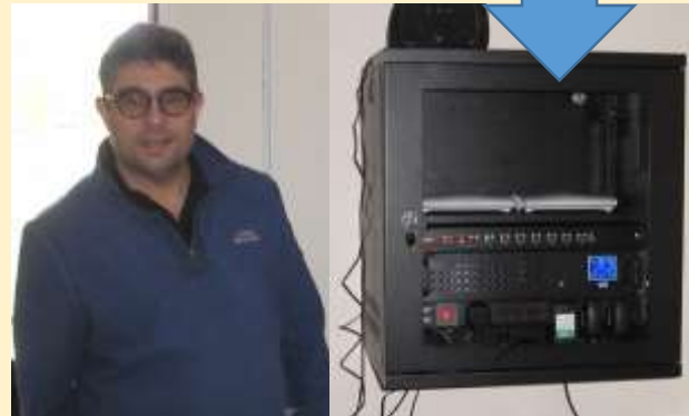
Mike Hicks from Cromarty Firth Wireless Networks installs the new cabinet at Stratherrick Hall.
