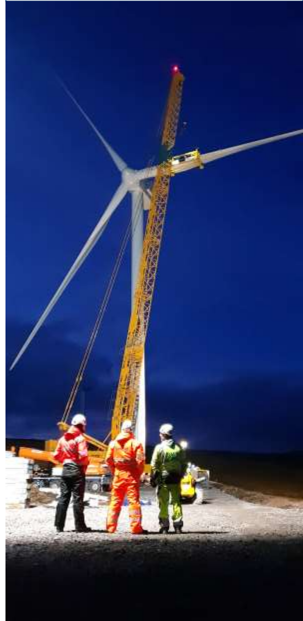
The final blade is fitted to the last of the 66 wind turbines at Stronelairg.
