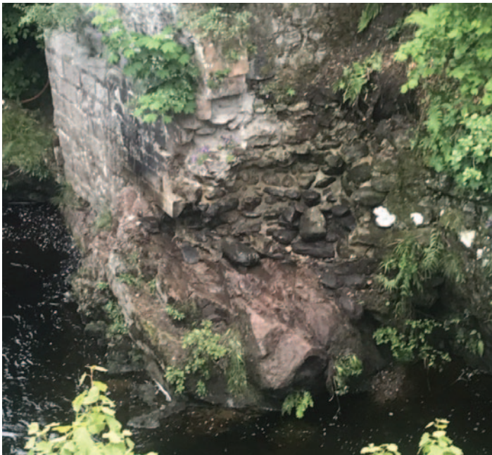
Eroded abutment before repair
